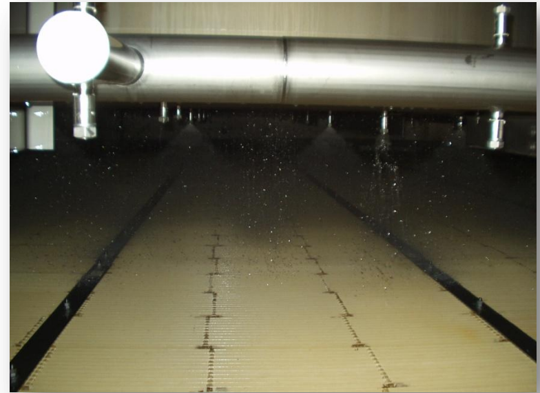
Mist Eliminator Wash System
